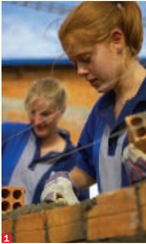
1: (left to right) New Collegians Pip Bowers and Madeline Sutton laying bricks.
