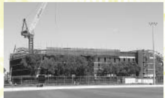
Construction of the fourth floor of New College viewed from the Village Green. Photo by Kwan Hee Lee.
